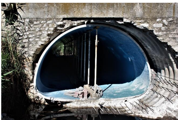
Figure 16c – GFRP pipes shored and buffered, ready to start the first stage of grout injection.
