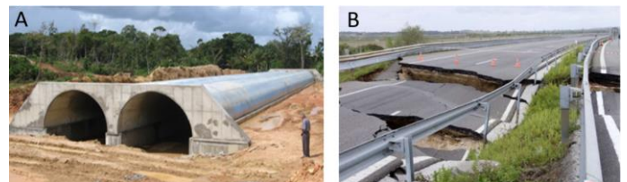
Figure 1 – a) Example of the ARMCO solution; b) Road subsidence in A41 (2016) Portugal [1].
